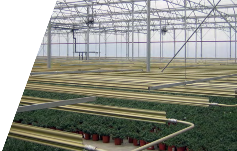
Aluminium greenhouse heating system
